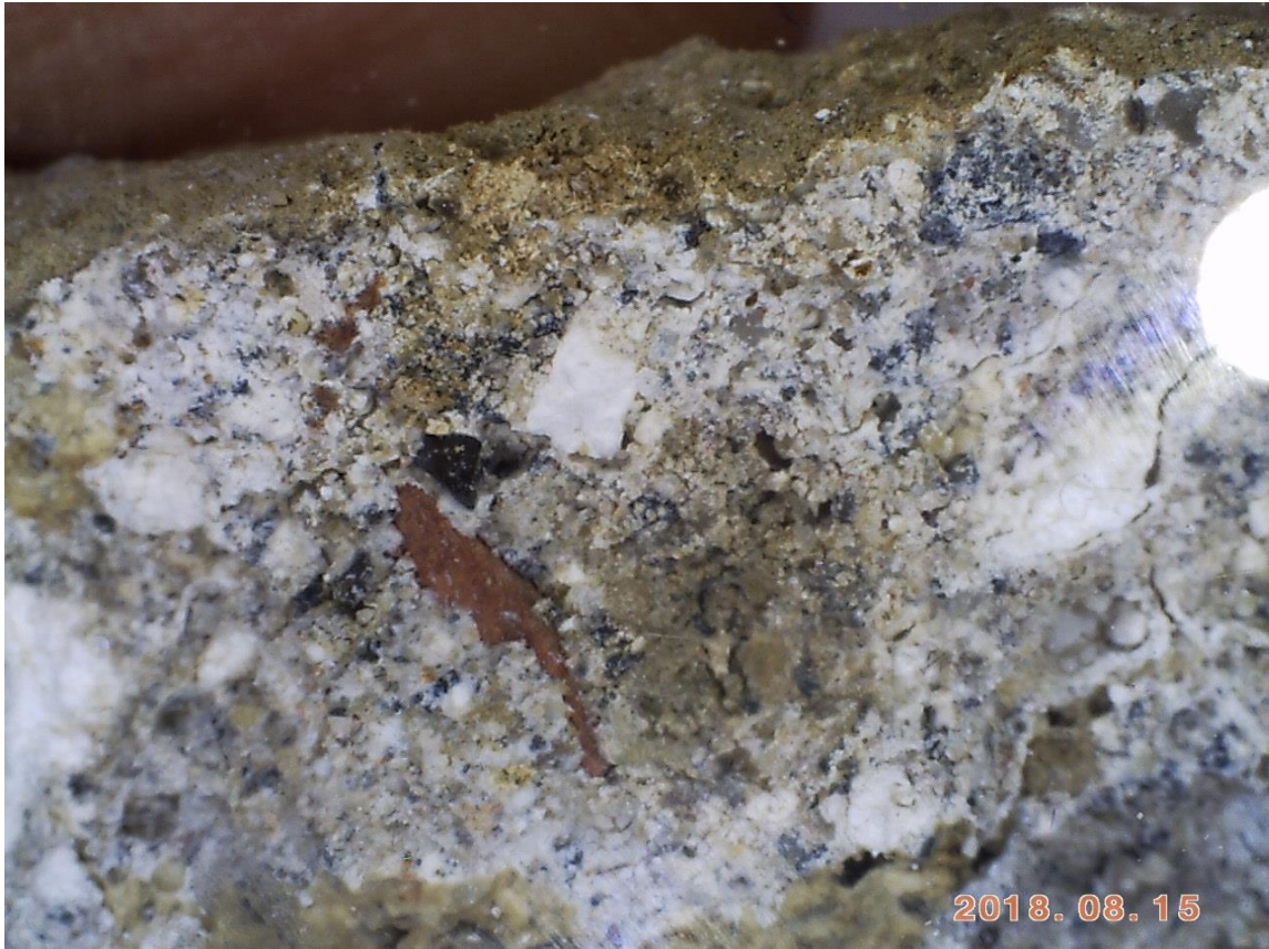
Above: Microscopic view of the mortar showing fine aggregate & an angular ceramic fragment (pozzolan, arrowed).
